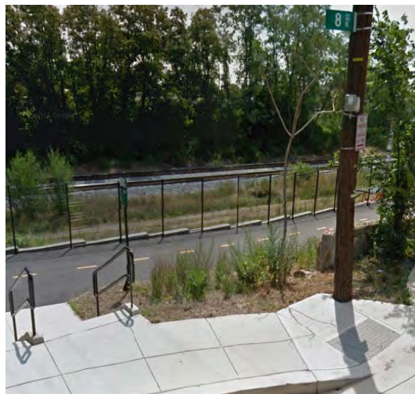
Figure 16 – Improper Pedestrian Ramp to MB Trail
